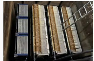
Turkey Waster Water Treatment
