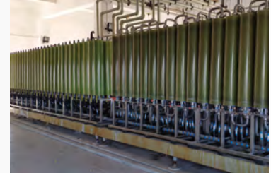
Guangdong Desulfurization Wastewater 48t/h
